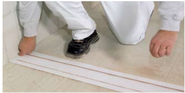
2. Repeat marking using chalk line on fixed MultiGips AkustikPro 120 s-a edge strip
